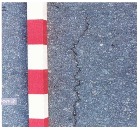
FIGURE 2.1. Fissure transversale : fissure franche et perceptible [LCPC, 1998]
