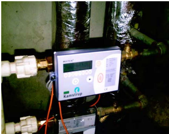
Figure 8-2 heat metres in a completed house
