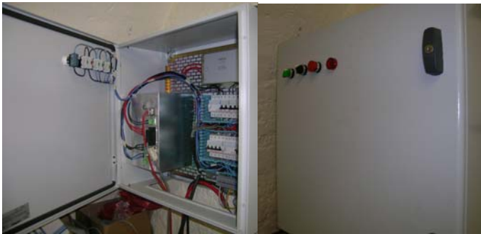
Electrical motor control box
