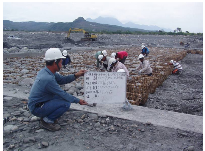
Fig. 2. Bamboo gabions currently used in Taiwan. (Photograph courtesy of Rui-Lin Chen, WRA Taiwan).
