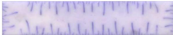
Figure 3.1: Crack pattern in a slab after a thermal shock [Jiang et al. 2012]
