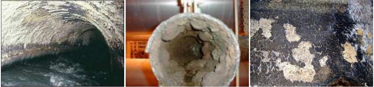
Figure 1.2: Examples of MICC of sewer pipe
