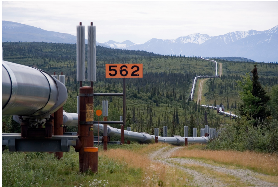
Figure I.15 – Pipeline Trans-Alaska muni de caloducs ailettés [7]
