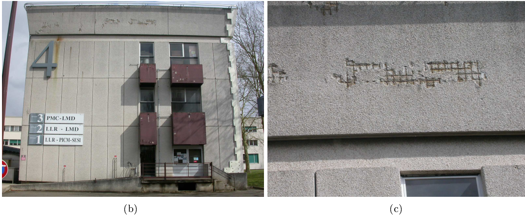
Figure 1.2: Carbonation. (a) Transport of the carbon dioxide gas inside the porous medium, (b) front of PMC Laboratory (c) zoom on the top of front of PMC Laboratory-cracks due to the corrosion of the structural steel.
