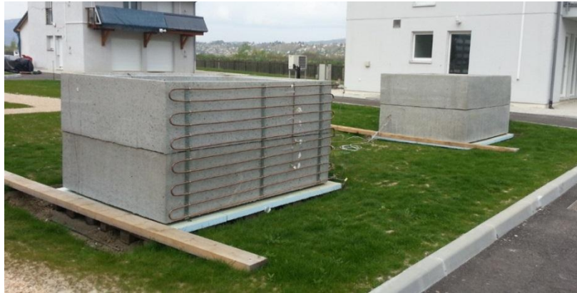
Fig. 3.21: The experimental mock-ups: the test-case with the fluid pipes and the reference case without the pipes (Note: this figure is before applying the coating on all the facades)
