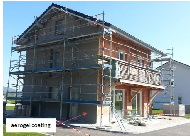
Fig. 3.13: The experimental test house while the aerogel-based coating being applied on its exterior facades
