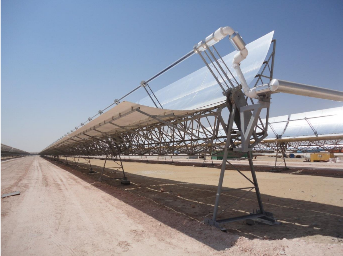
Fig. 1.1: Picture of the parabolic troughs of Shams 1, a CSTe power plant located in the UAE. © Yehia Eissa, 2012.
