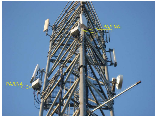
Figure 7.2: Antennas with PAs on mast
