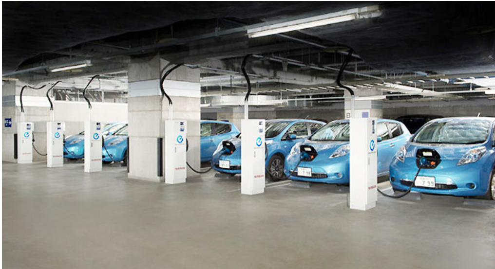
Figure 1.10: Vehicle-to-Building project. 6 Nissan LEAFs feeding an office building in Japan.
