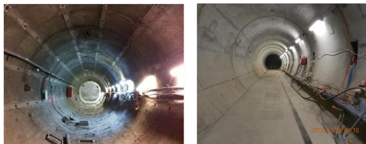
Fig. 2. 2. GCR section. Flexible support (left) and final lining installed after 7 months (right)
