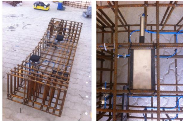
Fig. 1. 16. Implementation of measurements gadgets in the segments before the concrete is poured
