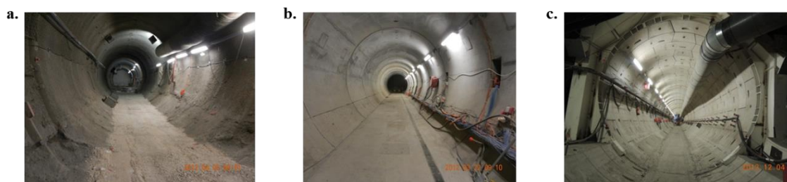
Fig. 1. 7. Rigid support installation: a. Support of 45 cm of fiber shotcrete (BEP drift). b. Support with 20 cm of fiber shotcrete and a permanent lining installation 7 months after (GCR drift). c. Support composed of rings of prefabricated segments (GRD4 drift)
