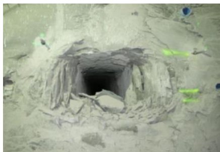
Fig. 2. 22. Induced fracture distribution around micro-tunnel ALC3005. It is observed the elliptical fracture distribution around the opening, with a larger extension in the horizontal direction. In the ascending vertical direction is observed the breakouts induced by the excavation
