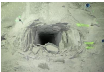
Fig. 2. 22. Induced fracture distribution around micro-tunnel ALC3005. It is observed the elliptical fracture distribution around the opening, with a larger extension in the horizontal direction. In the ascending vertical direction is observed the breakouts induced by the excavation
