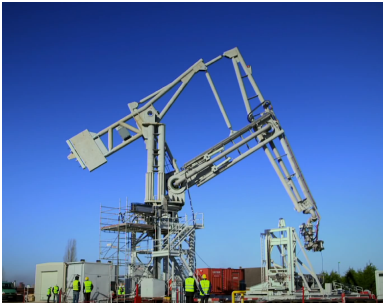
Figure 1.3: Offshore Loading Arm Footless (OLAF) - Prelude's loading arm.
