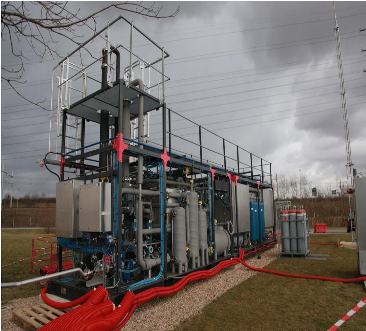
Fig. 29: BioGNVAL demonstrator located at Valenton water treatment plant [9]
