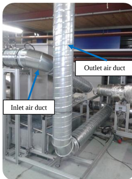
Fig. E.18: Air ducts
