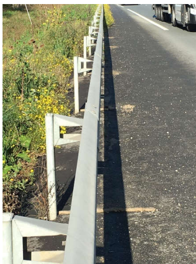
Figure 91 : Galvanized steel safety barrier separating the biofiltration swale from the road surface
