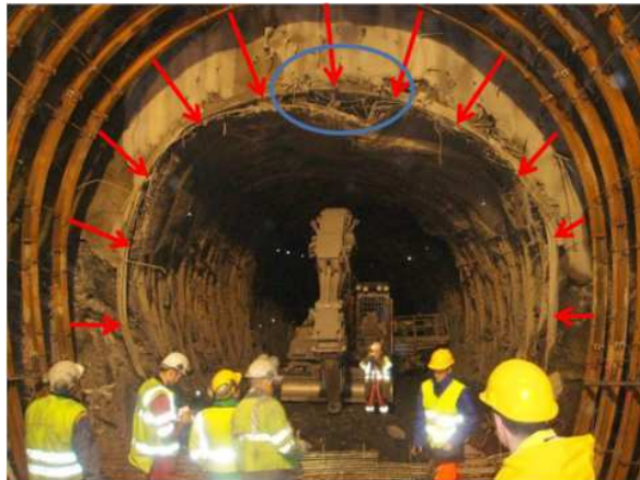
Fig. 1.8 Squeezing phenomenon in a cross section of Saint-Martin-La-Porte access adit (Lyon-Turin Base Tunnel), after Bonini & Barla (2012)
