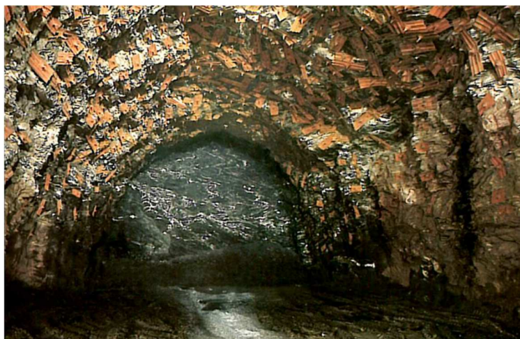
Fig. 5.5 Front face of the Fréjus road tunnel showing the support composed of rockbolts and a wire grid. Presence of schistosity planes at the tunnel face after SITAF (1982)
