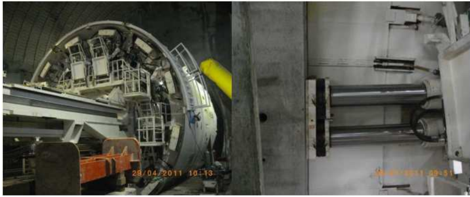
Fig. 6.3 Image of the hydraulic jacks of the TBM after Vinnac (2012)
