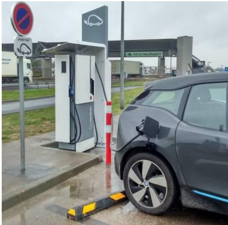
Figure 47 First station commercialized by the Consortium
