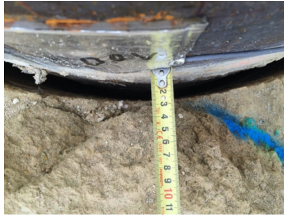
Figure 3.21.: Picture of the gap behind pile P2 after loading
