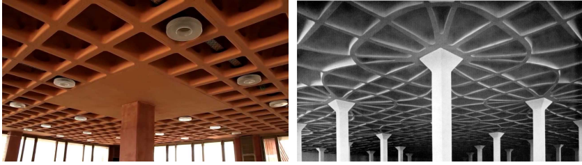
(a) Waffle slab without singularities (source: HOLEDECK) (b) Ribbed slab with singularities (source: Pier Luigi Nervi)
