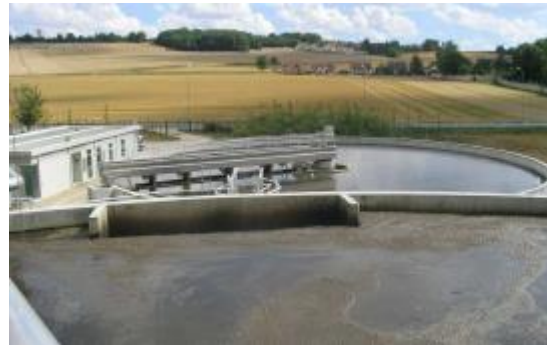
Activated sludge system (Provins, 23 330 PE)
