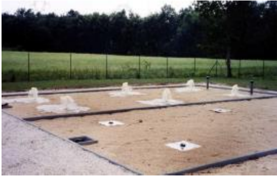
Sand filters (Forges, 110 PE)
