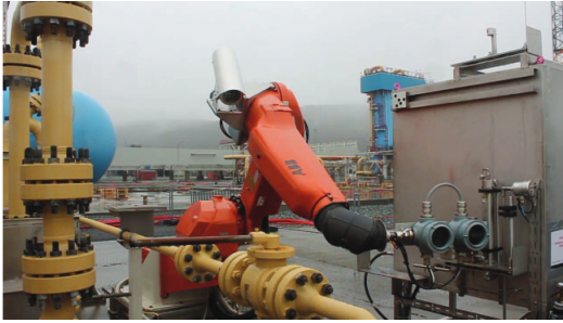
Figure 1.2: A robot operating in potentially explosive environment, among pipes carrying gas [4].
