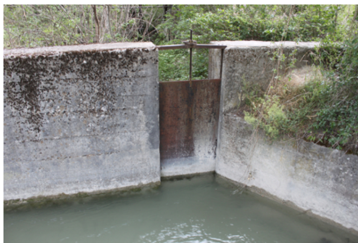
FIGURE 3.19: The floodgate of the water intake of the Aspres-Sur-Buëch gravity-fed network (credit : B. Richard).
