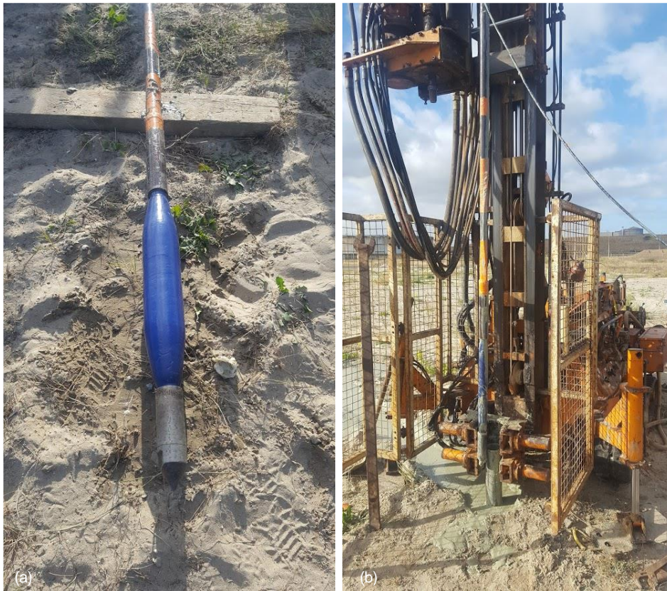
Figure 3.7 – (a) Photo of the probe assembled for the tests at Dunkirk site; (b) photo taken before probe insertion into the ground
