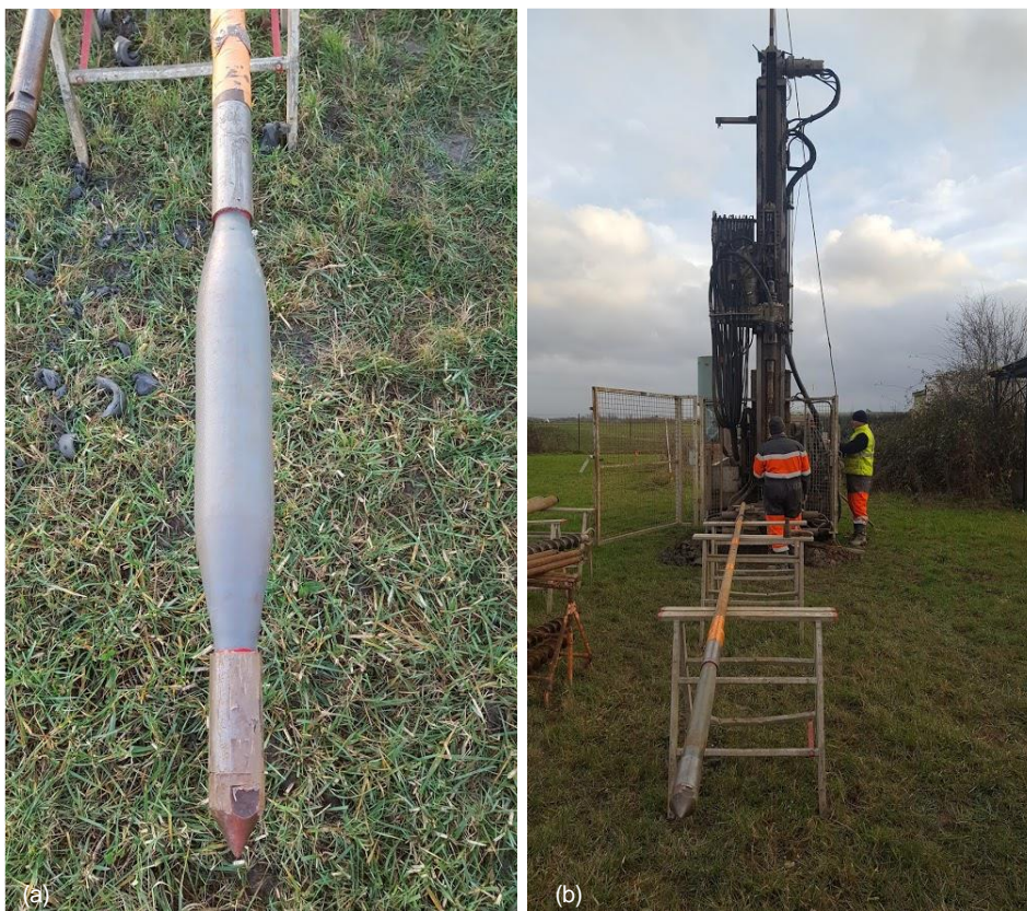
Figure 3.8 – (a) Photo of the probe assembled for the tests at Merville site; (b) view of the probe connected to the steel rods prior to its insertion into the ground
