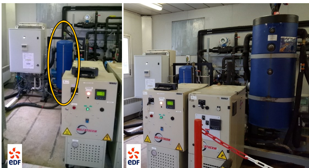
Figure 0-23: Cooling water unit platform
