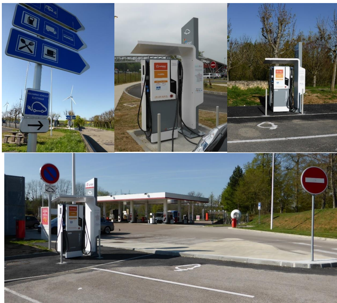
FIGURE 2-5 LA STATION DE RECHARGE CORRI-DOOR
