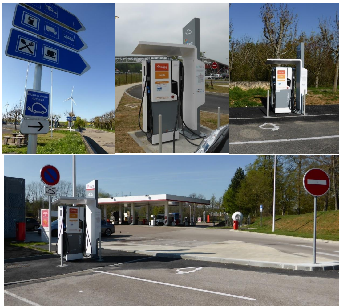
FIGURE 2-5 LA STATION DE RECHARGE CORRI-DOOR
