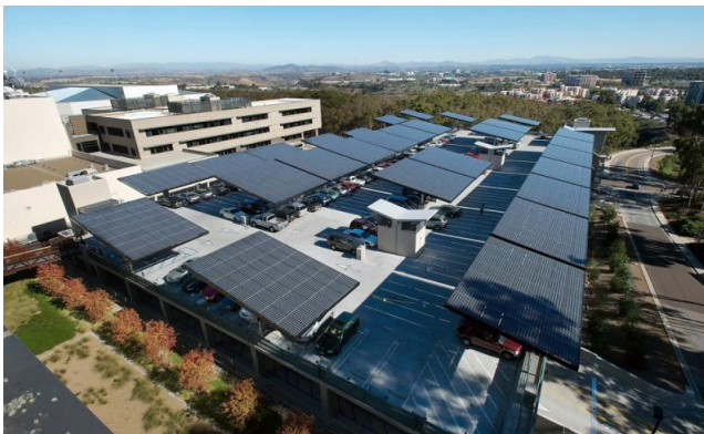
Figure 2.2: University of California San-Diego’s microgrid.
