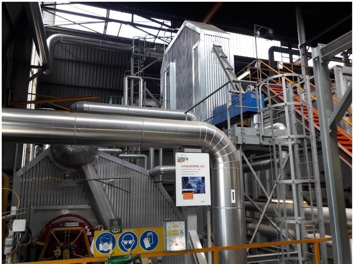
Picture 8 The explanatory signs for boiler G5
