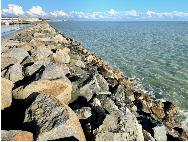
Figure 5.2: Photograph of an armoured rubble-mound breakwater (in La Pallice harbour, La Rochelle, France) similar to the model considered in the present study (photo: Hubert Branger).
