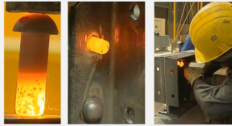
Figure 2.1 A rivet is heated, and inserted in the parts before its end is hammered. Renovations of the Grand Palais, Paris, France. Source: [1].
