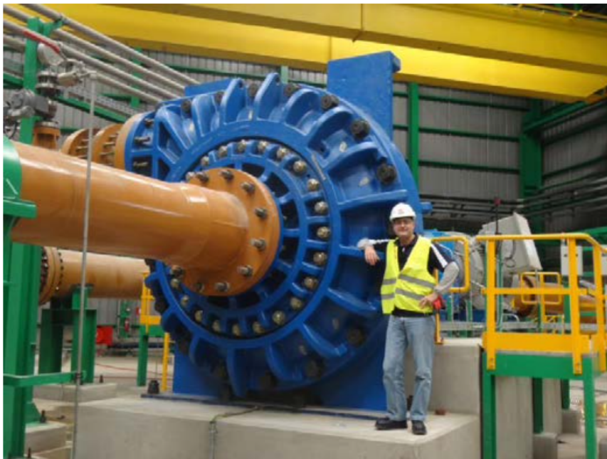
Figure 2.3: Head station slurry pump. Adopted from Rusconi et al. [2016]
