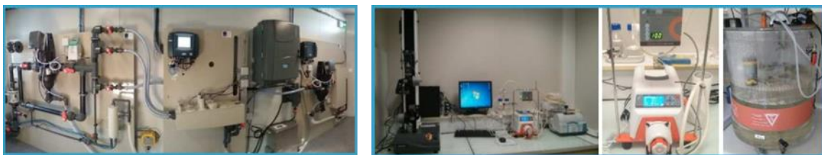
Figure 7: collection of real-time process data (left) supported by on-site laboratory analyses (right). (© SIAAP)
