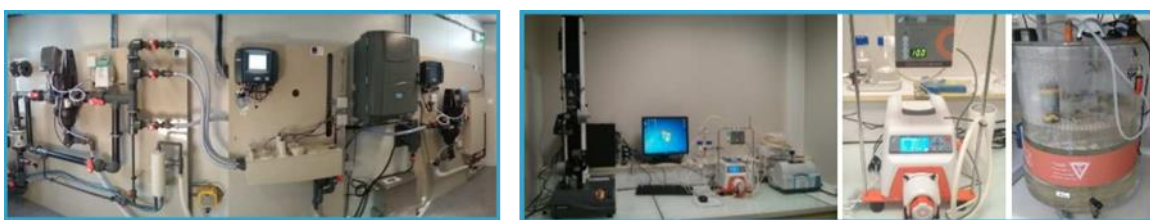
Figure 7: collection of real-time process data (left) supported by on-site laboratory analyses (right). (© SIAAP)
