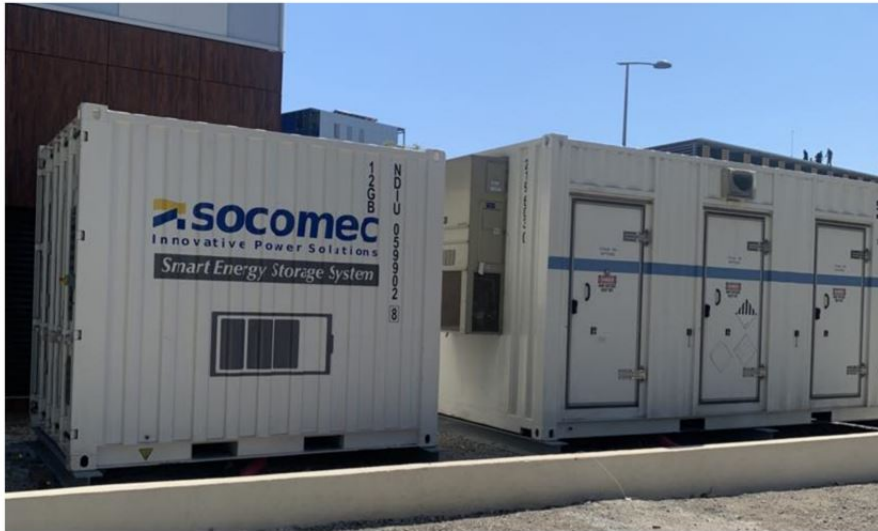
Figure 6.11: Picture of the battery energy storage system installed near to the power plant of the MSE eco-district.
