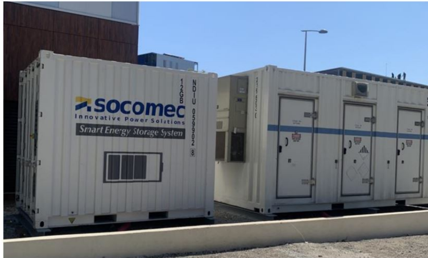
Figure 6.11: Picture of the battery energy storage system installed near to the power plant of the MSE eco-district.
