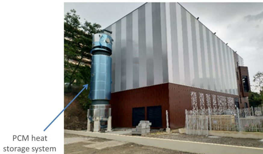
Figure 6.9: The PCM heat storage system of the MSE eco-district installed outside the power plant.
