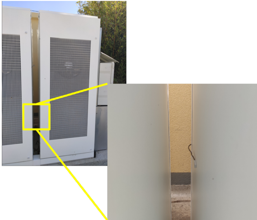
FIGURE 2.9 – Example of the temperature sensors installed outside the battery cabinets.
