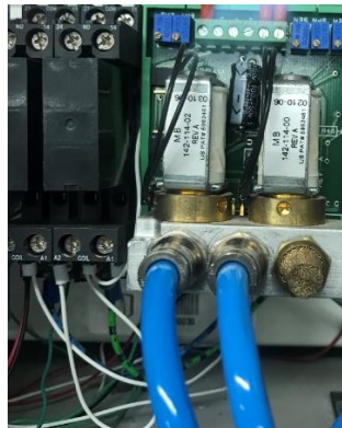
Figure 5-25. The Type 3110 Bellofram transducer was used to control the air pressure acting on the jack.
